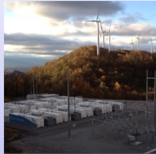
AES Energy Storage Laurel Mountain
